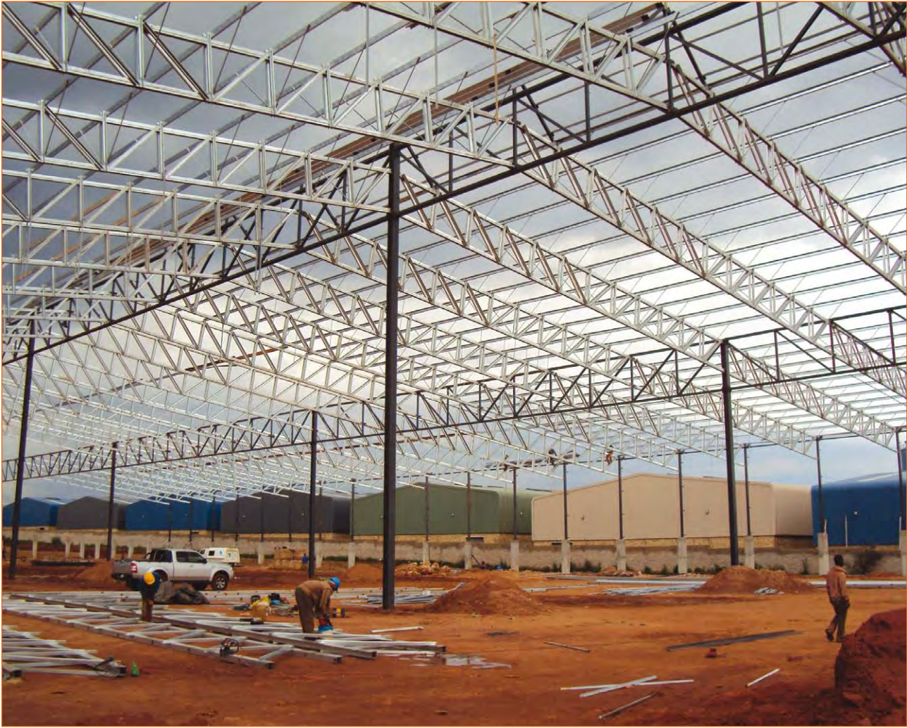
Eureka used Robor's innovative Hybrid Structure for constructing its 11 800m 2 DIY factory in Gauteng. The structural steel is lightweight and allows for customisation.
